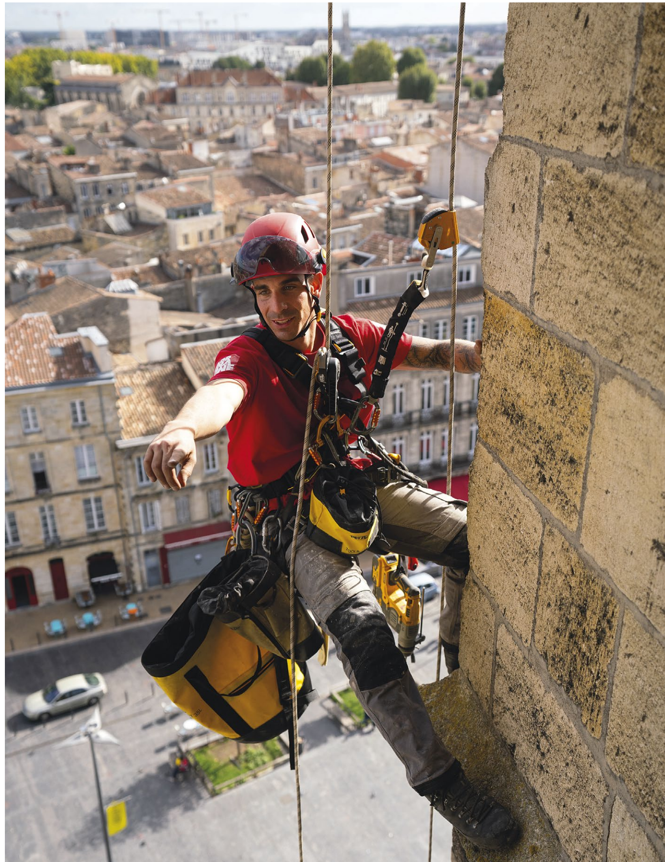
Installing monitors on the spire of the St Michel Church, Bordeaux, France © 2021 Petzl Distribution - Vuedici.org - Adrénaïne - Bordeaux City Hall
