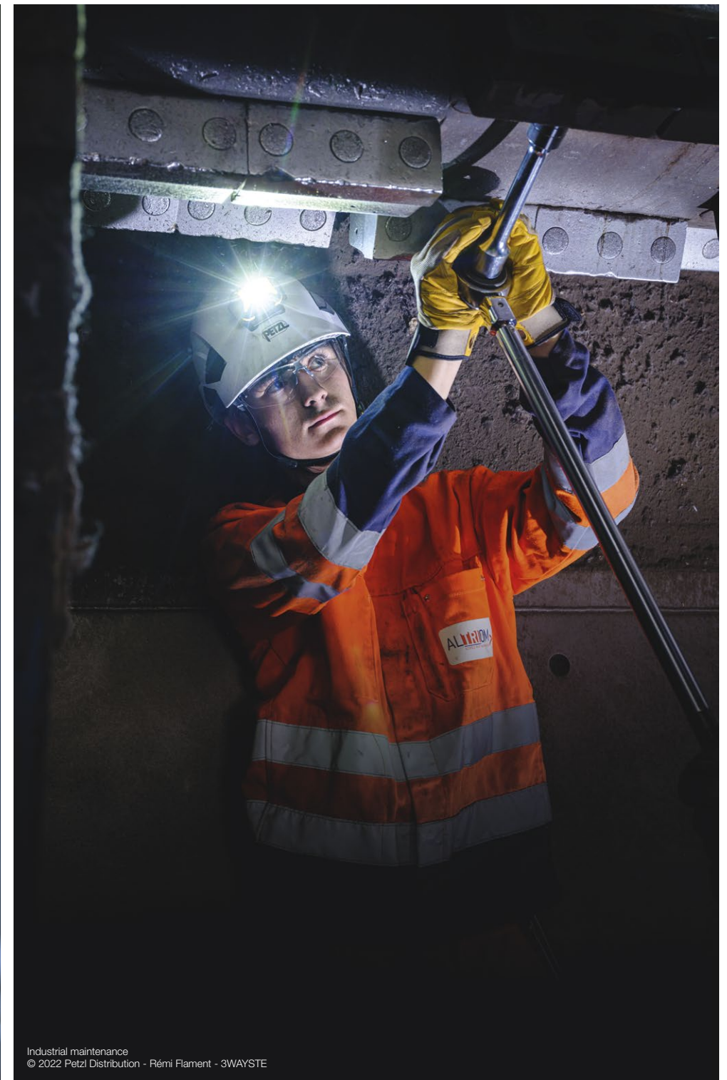
Installing monitors on the spire of the St Michel Church, Bordeaux, France © 2021 Petzl Distribution - Vuedici.org - Adréline - Bordeaux City Hall
