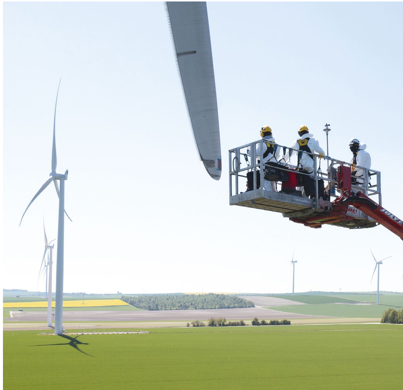
Wind turbine maintenance © 2022 Petzl Distribution - Vuedici.org - GR Wind - Vestas - Joly - EDF Renewables - Les Coteaux wind farm
