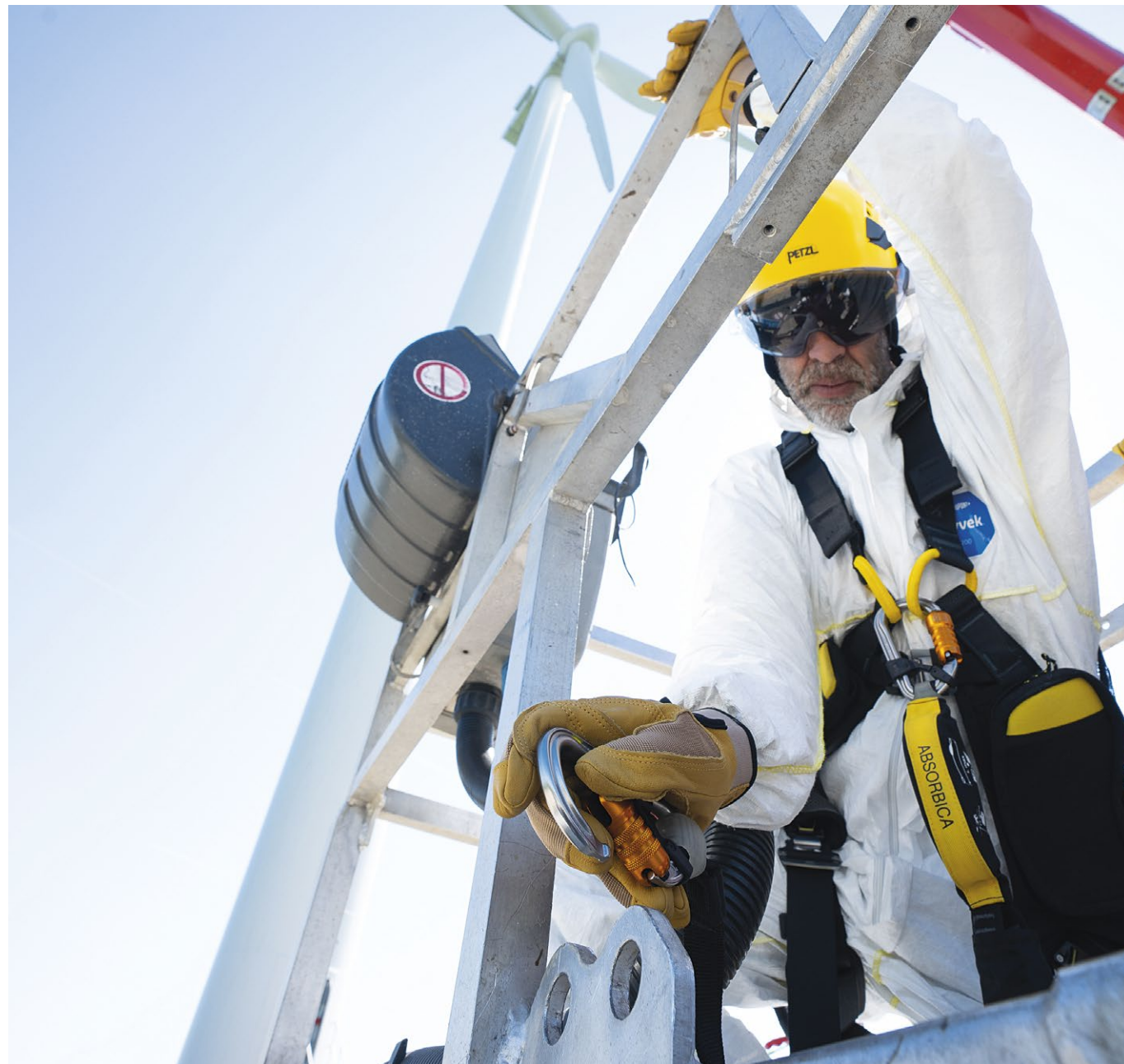
Wind turbine maintenance © 2022 Petzl Distribution - Vuedici.org - GR Wind - Vestas - Joly - EDF Renewables - Les Coteaux wind farm
