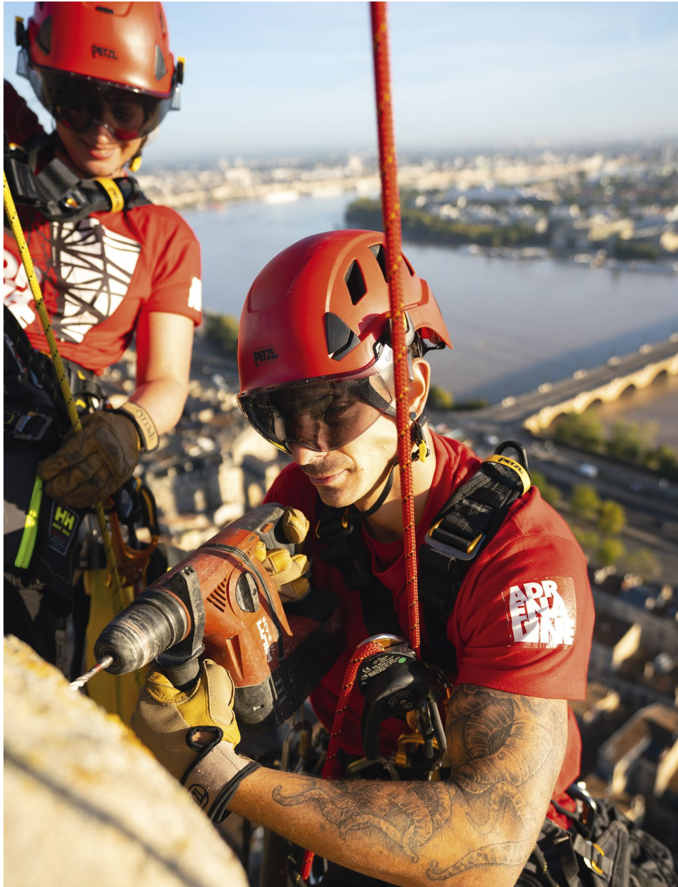
Installing monitors on the spire of the St Michel Church, Bordeaux, France © 2021 Petzl Distribution - Vuedici.org - Adrénaïne - Bordeaux City Hall
